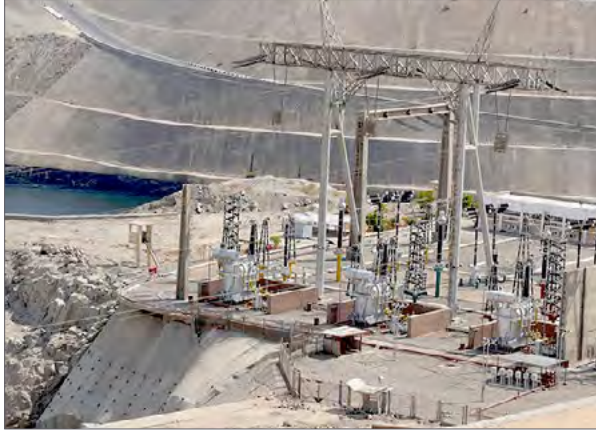
Aswan Dam hydroelectric power plant, Upper Egypt Wikimedia/Ad Meskens/CC BY SA 3.0
