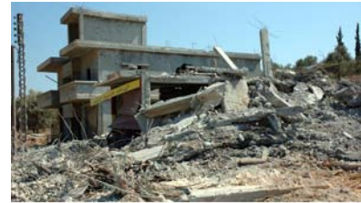
© Julien Harnais Earthquake damage
