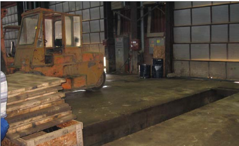
Oil Slump and Inspection Pit © Lee Bryant
