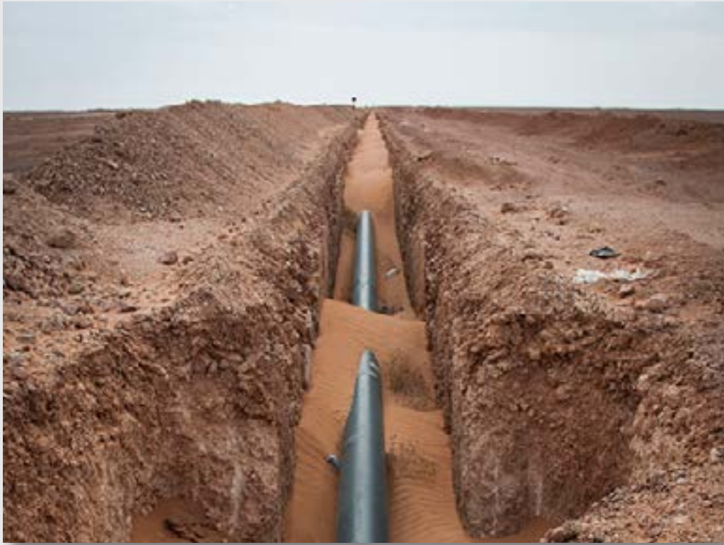
Building gas pipe Flickr / iñaki do Campo Gan
