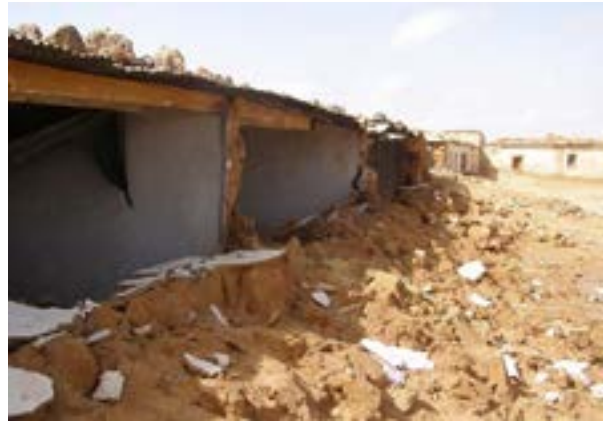
Damages caused by flooding, Algeria Flickr / Western Sahara
