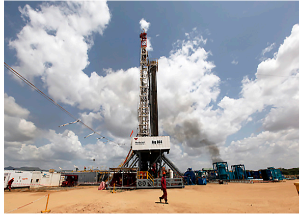
A worker and an oil rig in Turkana County, Lokichar Basin Flickr / DEMOSH
