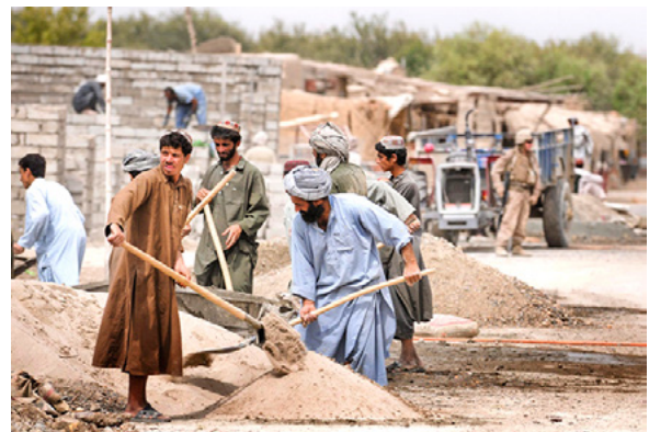
Afghans constructing new buildings which will expand the bazaar in the Nawa District of Helmand Province Flickr/ResoluteSupportMedia
