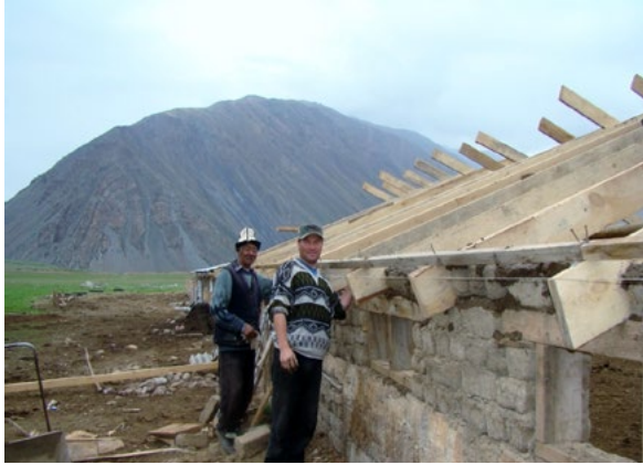
Repairing a sheep yard in the village of Kyzyl-Oj, Naryn Flickr / UNDP in Europe and Central Asia
