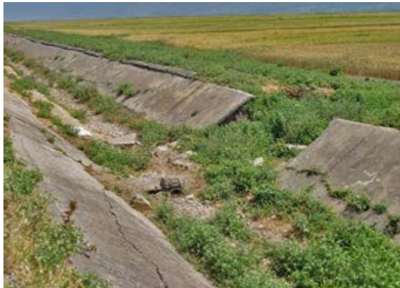
Damaged irrigation canal, Ghab Valley Flickr / Water Alternatives
